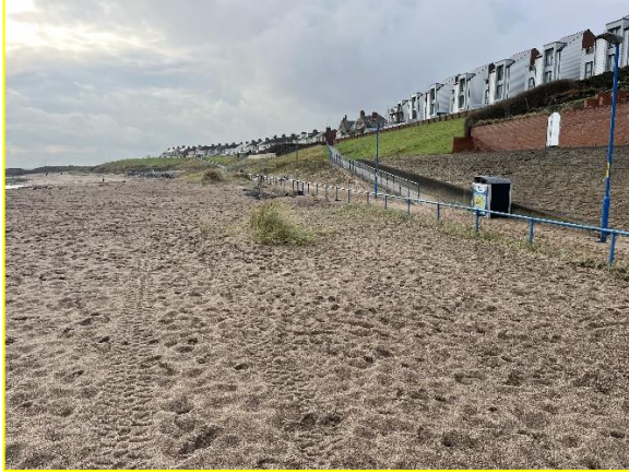
Rock armour, in parts, entirely buried by high beach levels (/3601C08)
