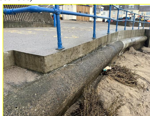
Loss of sealant at joint with existing seawall (/3601C06)
