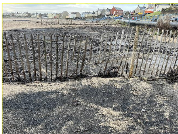
Minor damage to picket fencing but overall, in good condition (/3601C06)
