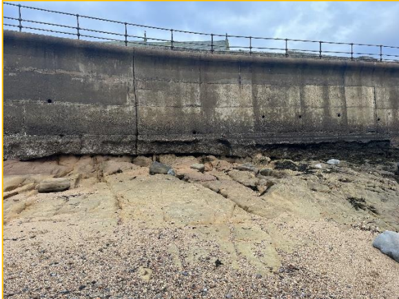
Church Point seawall in fair overall condition with localised undermining of toe protection (/3601C12)
