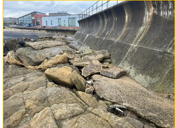
Concrete apron of recurved wall in poor condition (/3601C13)
