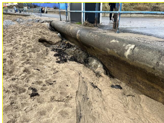
Exposed geotextile adjacent to slipway (/3601C06)
